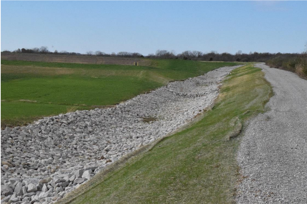
Closed ash pond – interior
