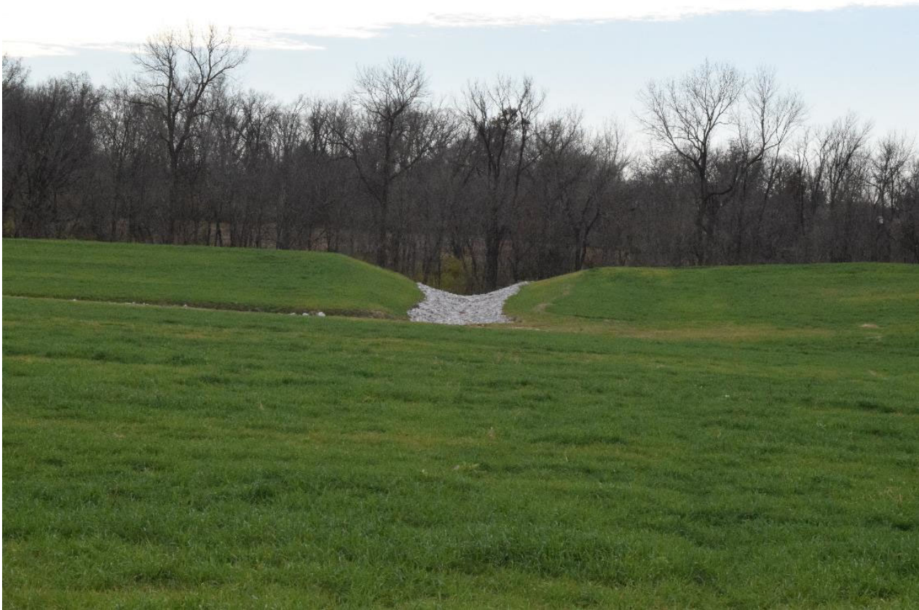
Closed ash pond – interior
